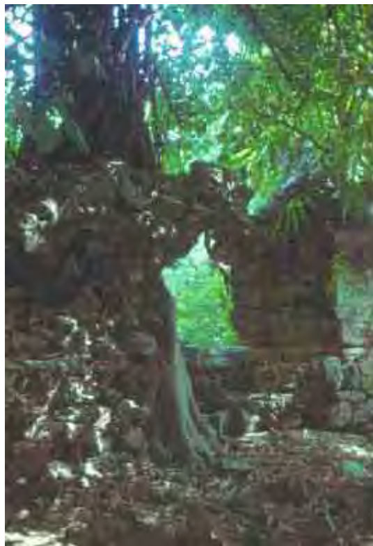
Through negligence ‘a stone wall is broken down’
